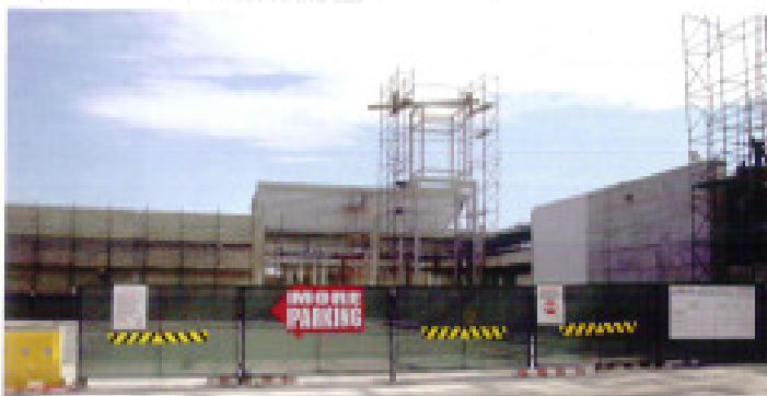
The Glen shopping centre extension project has been challenging and technical and is being done on an operating shopping centre.
